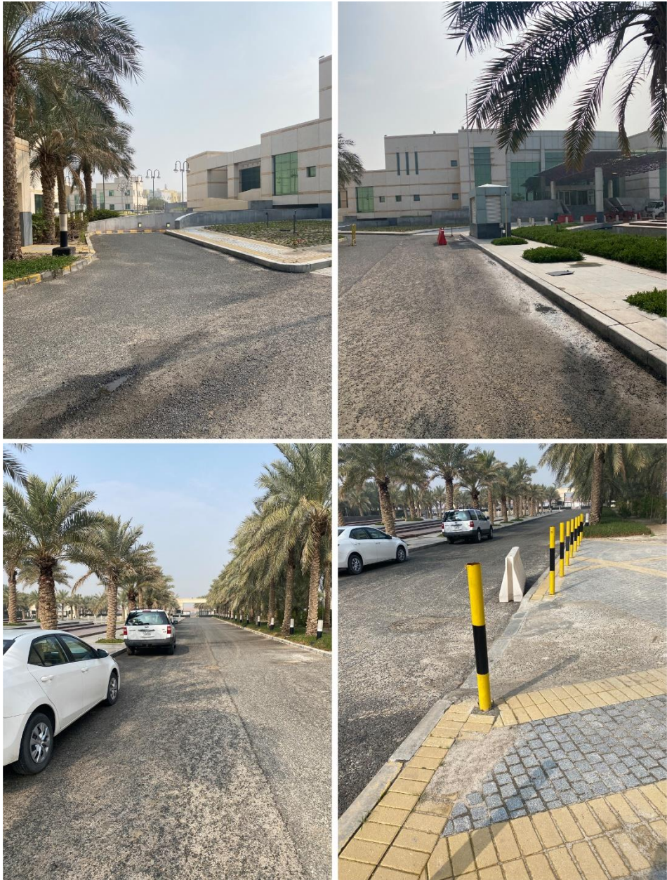
(Figure 1) Images of the linkage between the roads and the sidewalk. (Images by the author)
