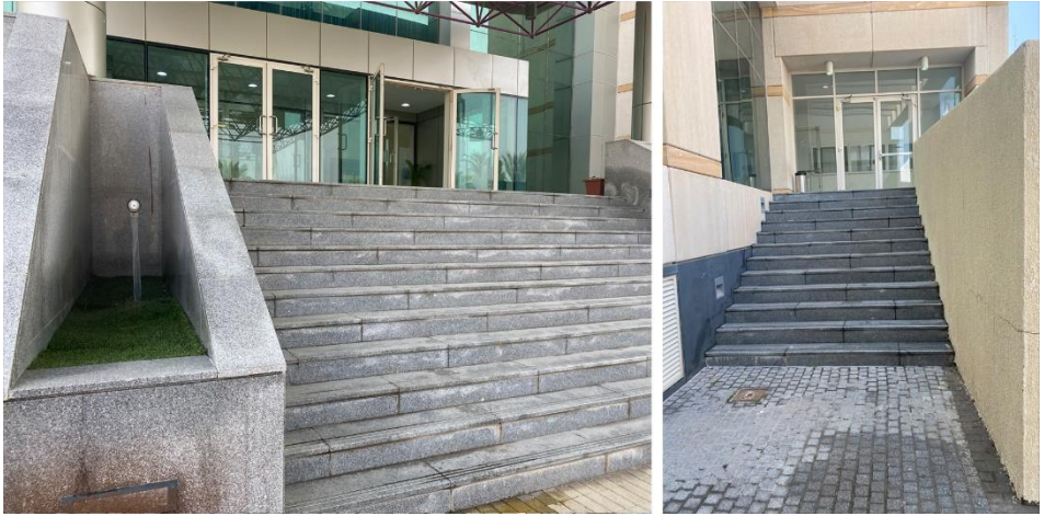
(Figure 5) Images of main entrance staircases. (Images by Author)
